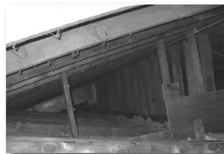
Joists and rafters and insulation above the hall stage. If you look closely at the top right, you see the cord that connects to the wood block and pulley system for the "disco ball"!
