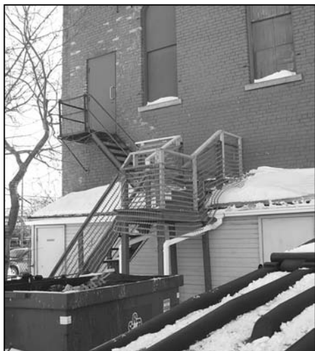
Above: Temporary remediation of fire escape citation, 2/1/2014
