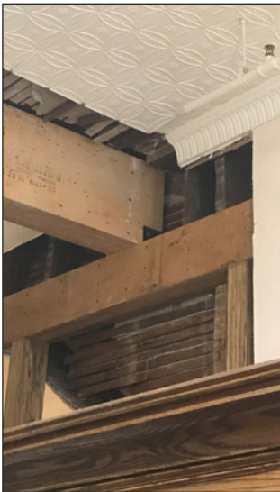
New structural support beam under the main stairs to the second floor
