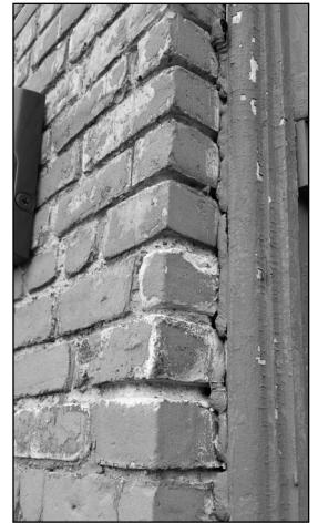
C.S.P.S. Hall brickwork needs tuck pointing
